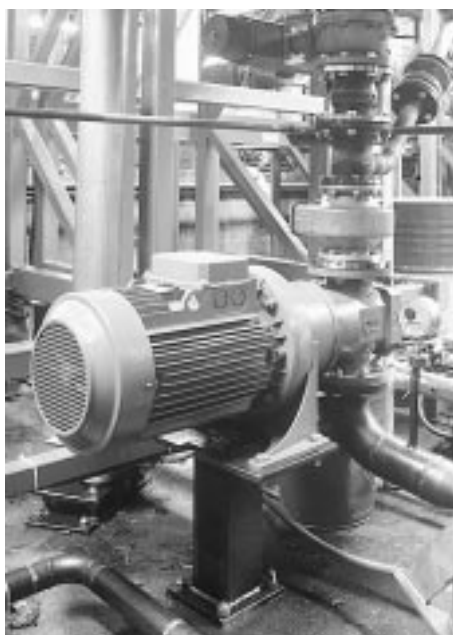
Fig. 12 Pump handling additives for lube oil production.
